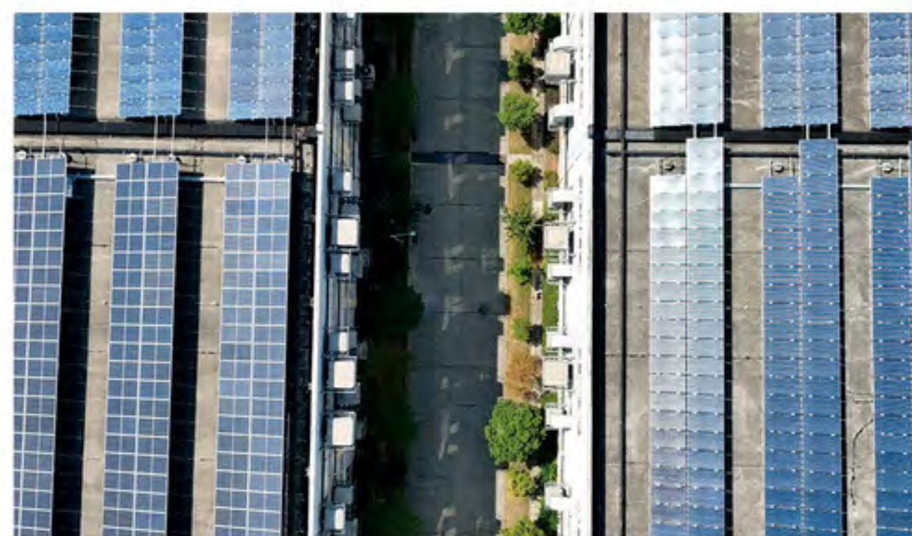
Industrial Rooftop Solar Panels
