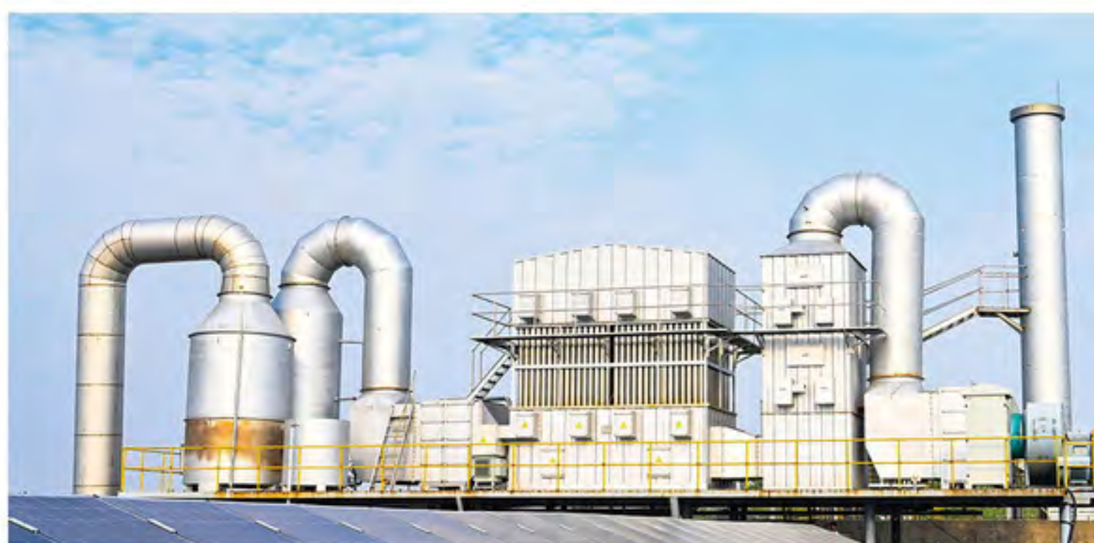
Exhaust Gas Treatment System
