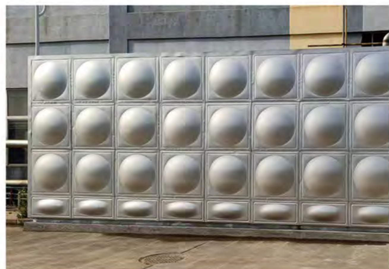
Waste Heat Recovery and Reuse System
